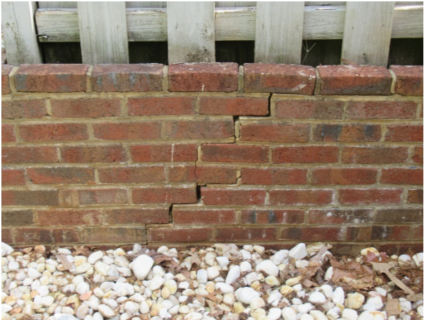
Masonry retaining wall step cracks
