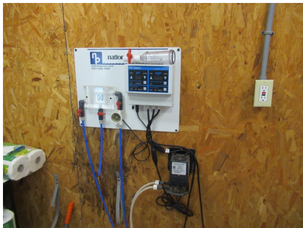
Mechanical equipment overview
