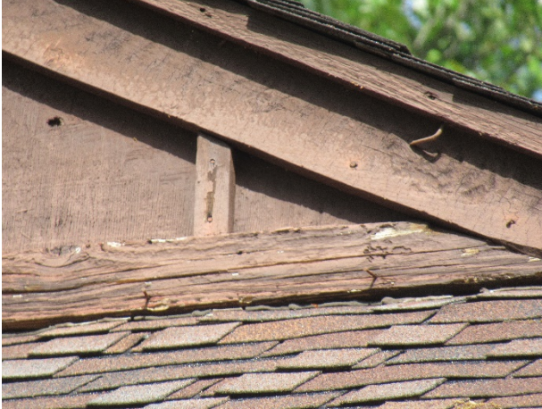
Wood trim deterioration
