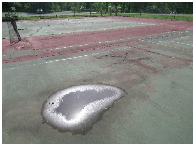
Cracks and evidence of standing water
