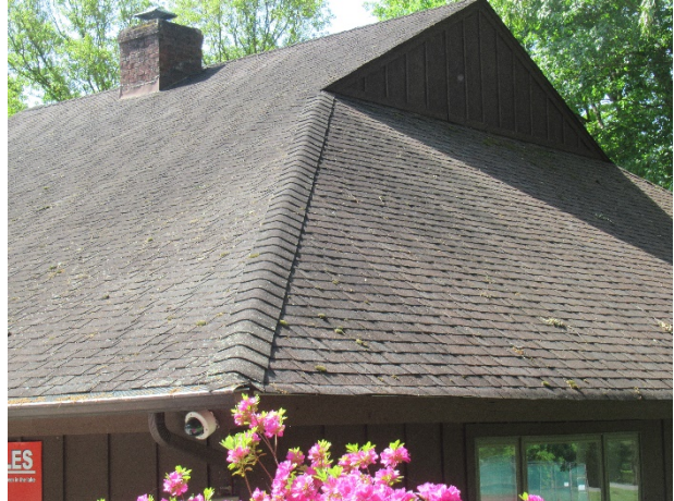
Clubhouse roof overview – Note: organic growth
