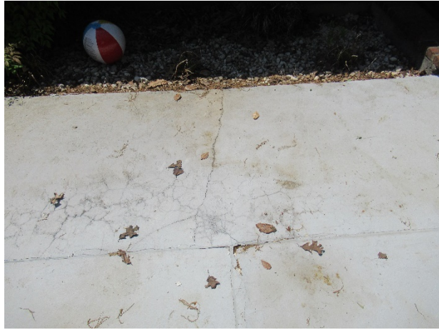
Concrete deck cracks
