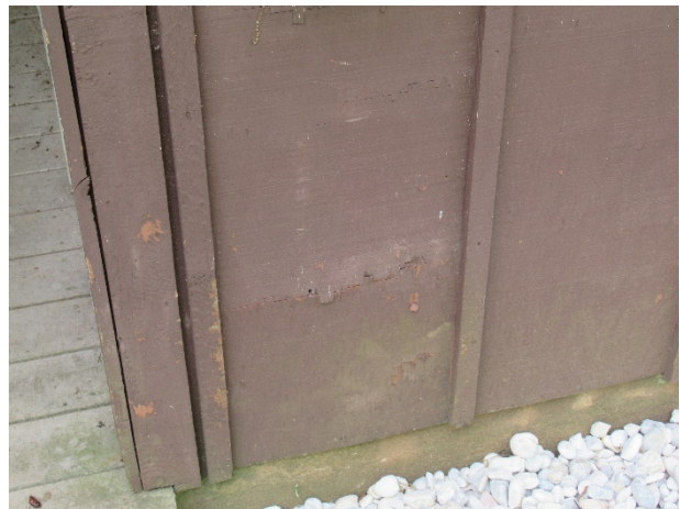
Wood siding finish deterioration
