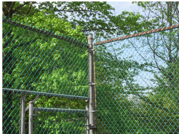
Rust at fence
