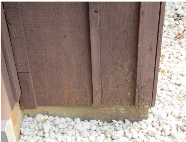
Wood siding finish deterioration
