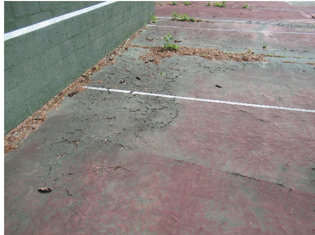
Cracks and deterioration
