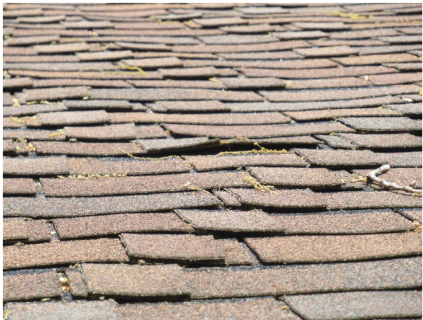
Clubhouse roof shingle lift and organic growth
